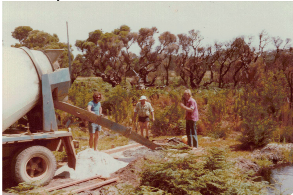
1980 Preston and Jim House, with Dereck Trigwell, putting down the foundations for the first pump between 5 and 7.
