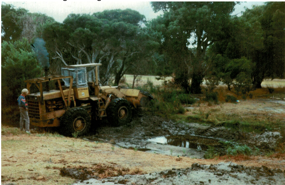
1981 Putting in the water hole at the front of 9 tee Leith Shepherdson
