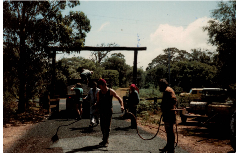
1985 The sealing started at the front entrance (note the original gate). Ray Atcheson organised the working party and all materials.
